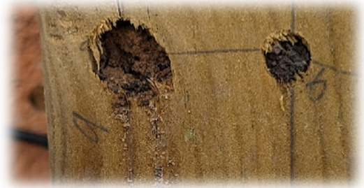
Rain damage to mud-capped tubes
